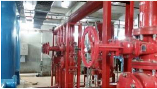
Fire Suppression & Fire Fighting Package PT Berca Hardayaperkasa Phase 1 Site Data Center Indokeppel
