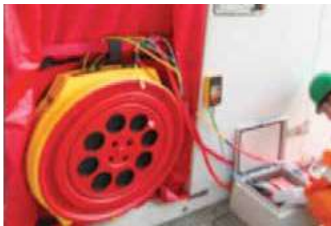
Room Integrity Test Gas Turbine BP Tangguh
