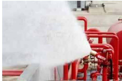
Foam System Package Smart Refinery-Tarjun
