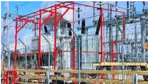
Fire Protection Package PT. PP (Persero) Tbk - Portsite Dual Fuel Power Plant PT Freeport
