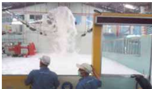
High Expansion Foam System Gajah Tunggal Tire Factory-Tangerang
