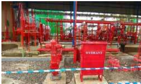
Fire Protection Package Indonesia Power, PLTU Holtekam Jayapura
